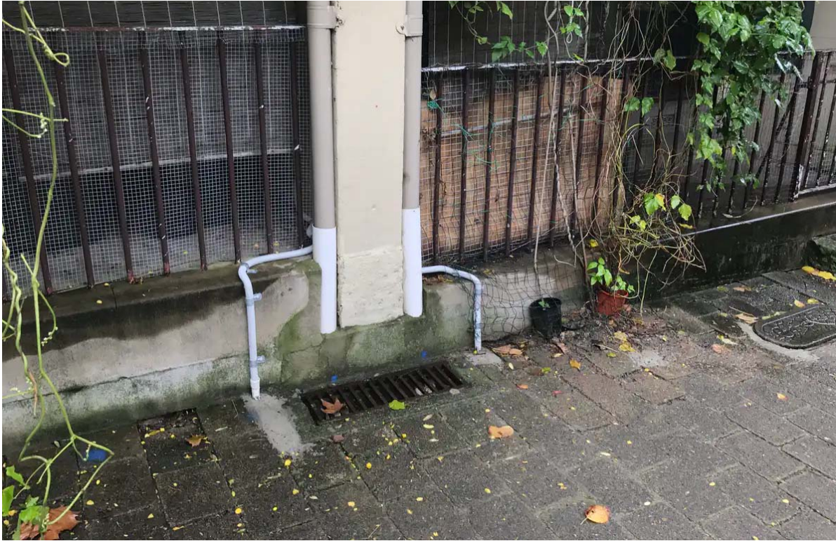
One heritage-listed house with two NBN installations (Judge Street, Woollahroo, NSW). Image: Stacey Miers, Author provided
