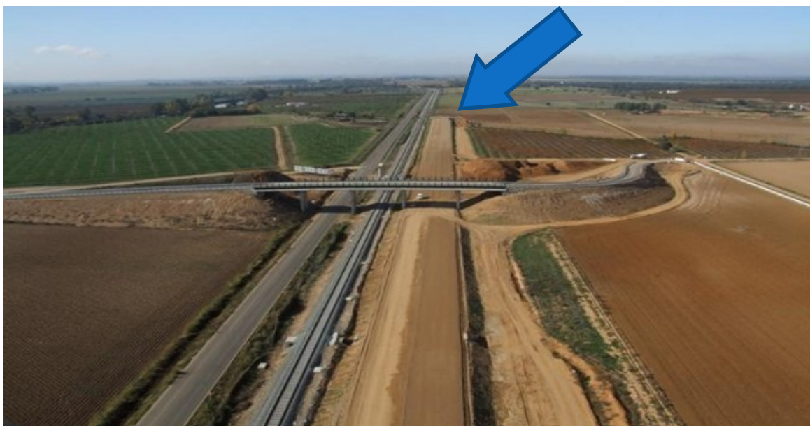
Picture 1 - Missing link at the border crossing on the Madrid-Lisbon high-speed line
