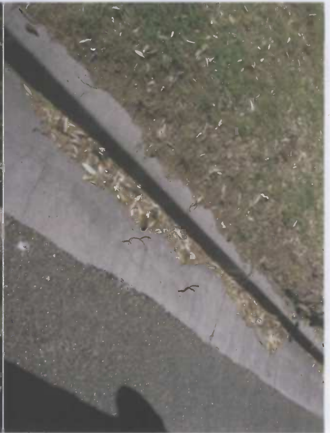
Photograph (3) Ronald Avenue Street Kerb ( Kerb Detail Next To Street Tree To Be Retained )
