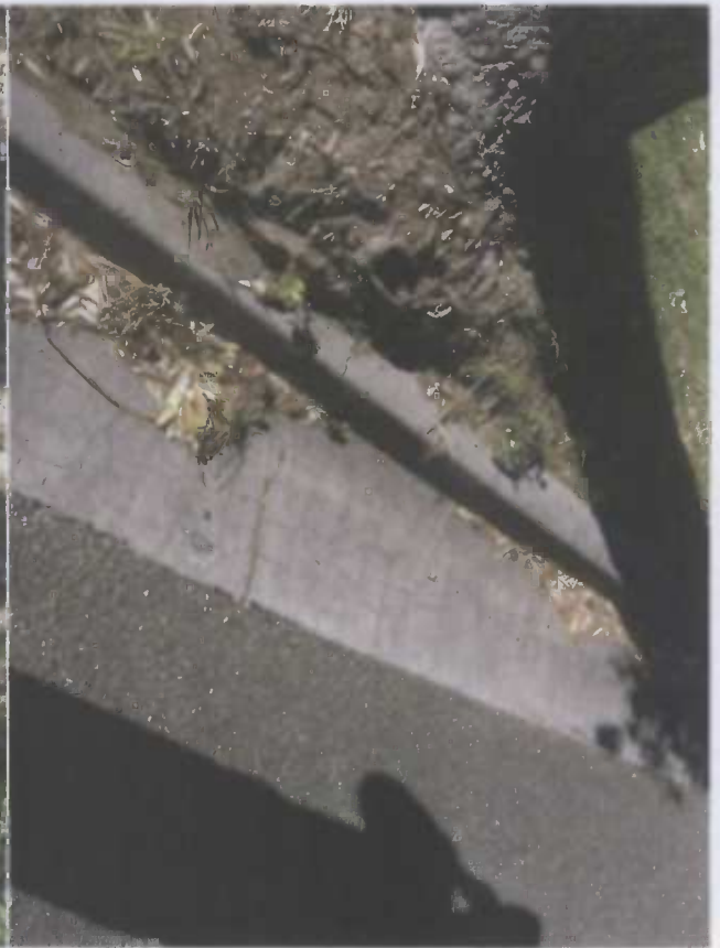
Photograph (4) Ronald Avenue Street Kerb (Kerb Detail Next To Street Tree To Be Removed )
