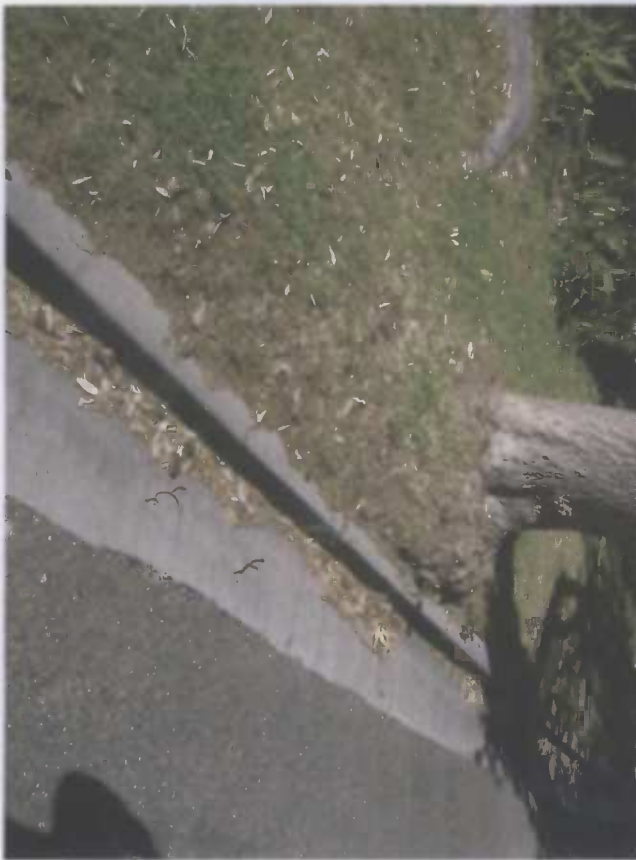
Photograph (2) Ronald Avenue Street Kerb ( Kerb Detail Next To Street Tree To Be Retained )
