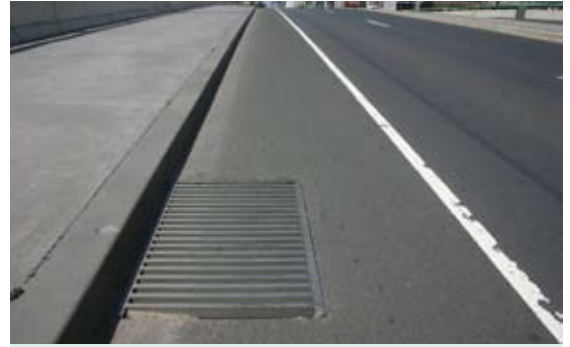
Figure 3 – Drainage grate with perpendicular bars in bicycle lane on La Trobe Street, Melbourne
