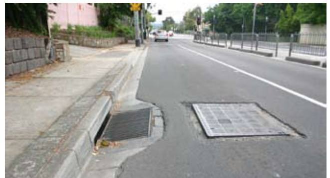
Figure 2 – The groove to the left of this pit lid is in the travel line for cyclists and poses a serious risk
